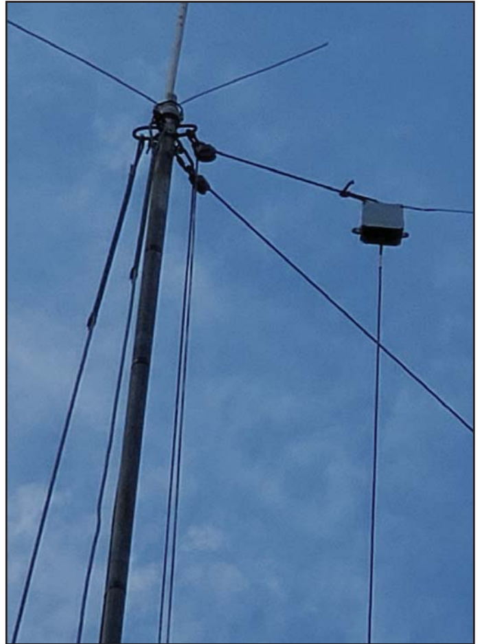
Photo D. Unun installed on an end-fed antenna
